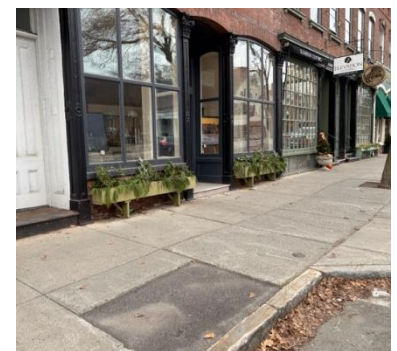
One of several filled-in tree wells on Central St. where we'd like to plant a tree.
